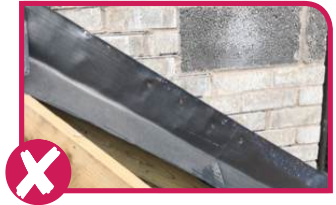
Photo 2 – Flashing not linking to cavity trays
